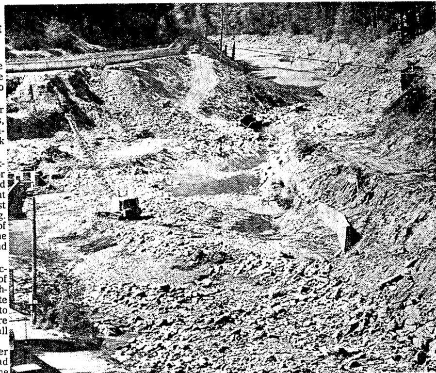
REPAIR WORK continues on Portland General Electric Co.'s Cascadero Dam, located three miles above Estacada on the
